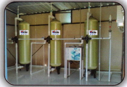
Nitrate/Arsenic/Iron removal plant
