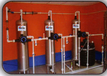
HAIX-Nano Fluoride Removal plant
