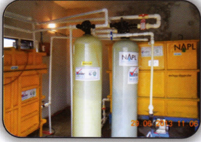
Electrolytic De-fluoridation plant
