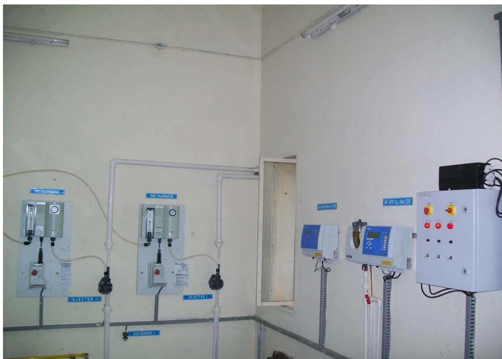
Auto Chlorination & Chemical Feed System
