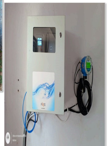
Residual chlorine analyzer
