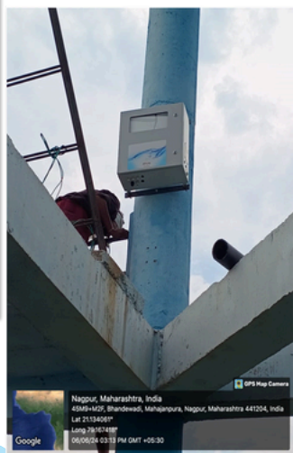
Residual chlorine analyzer
