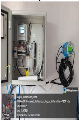
Residual chlorine analyzer
